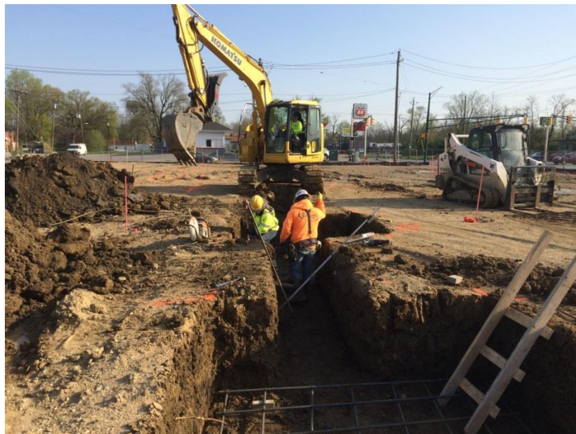
Project Site on April 23, 2019 View of the Exterior Wall Footing Excavation and Concrete Forming.
